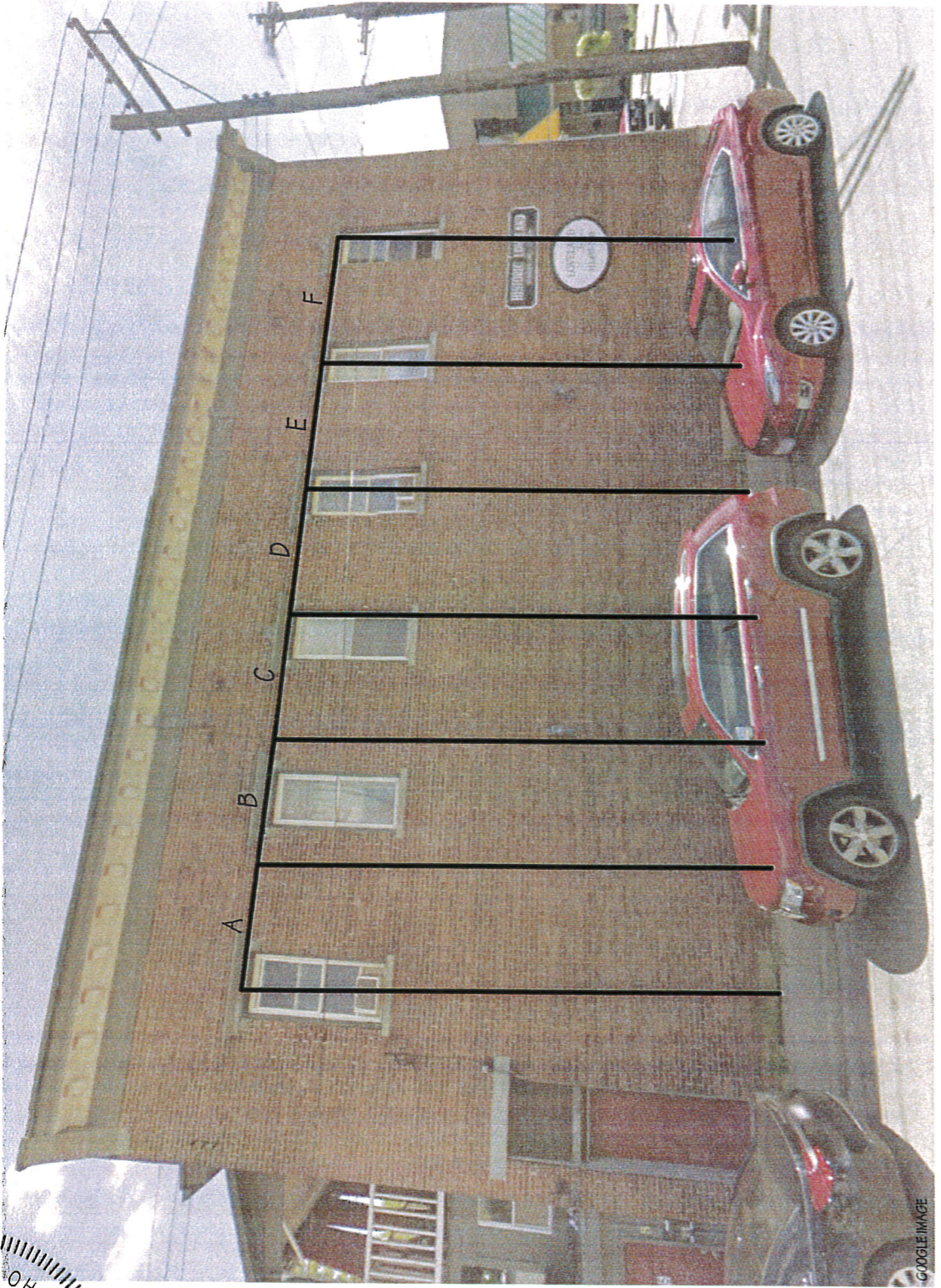
KARL BROWN WAY LOOKING EAST NOT TO SCALE (ONLY POSTS NEXT TO WALL ARE SHOWN)
